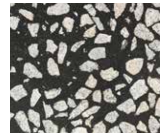
ASPHALTE PONCE INSERTIONS GRANIT (sol hall, sol parvis sud, sol parvis nord)
